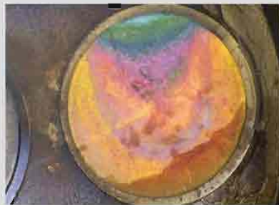
THIS IS a very sick exhaust valve on the verge of failing catastrophically. Note the asymmetrical appearance: That's bad!
