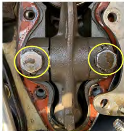
LOOSE ROCKER SHAFT bolts in this cellphone photo were noticed by Tony.
